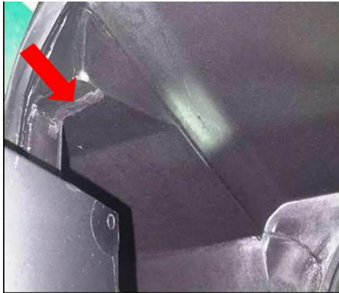
Fig. 3 Plastic Rib Removed
